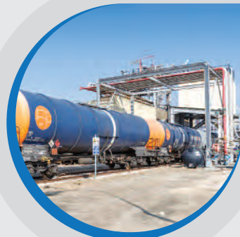
Rail car loading stations
