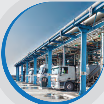
Truck loading stations
