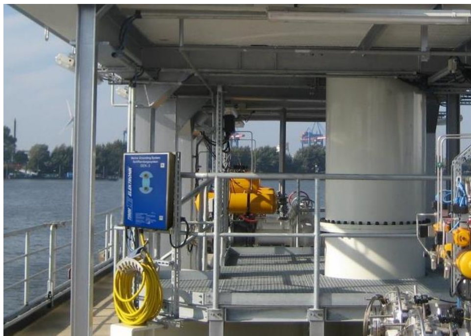
Control Device installed at jetty / pier
